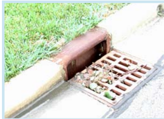
Debris accumulated on a storm sewer grate
